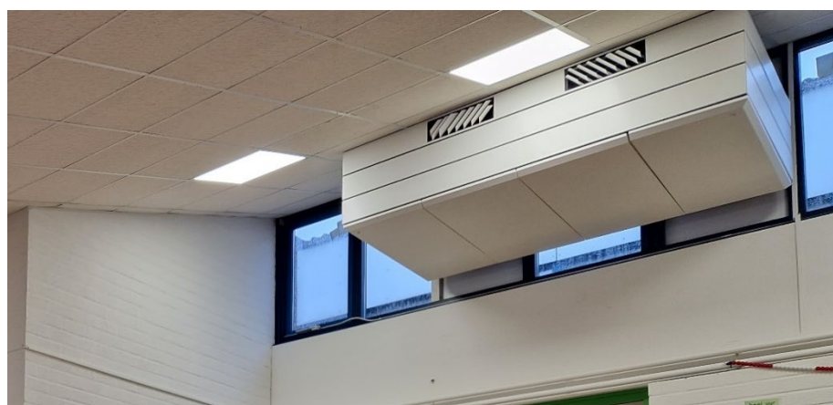
Figure 3-1 – Ventilation system after intervention
