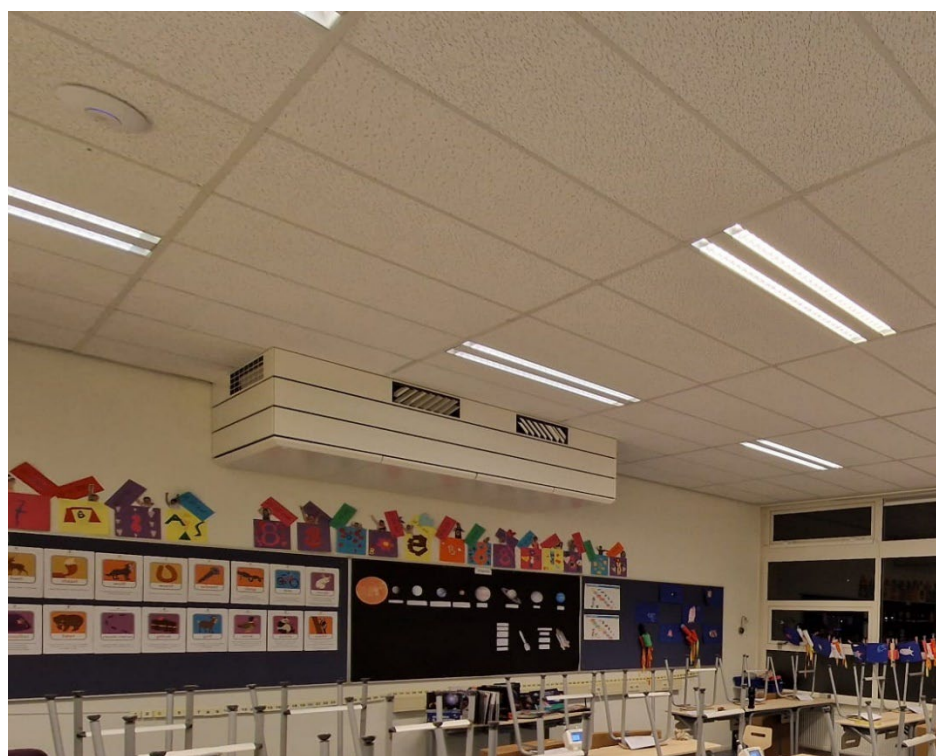
Figure 3-1 – Ventilation system after intervention
