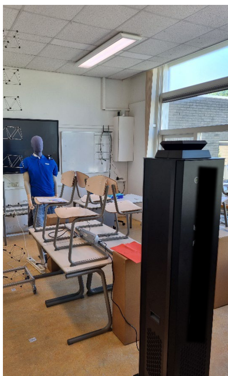
Figure 3-1 – Ventilation system after intervention A
