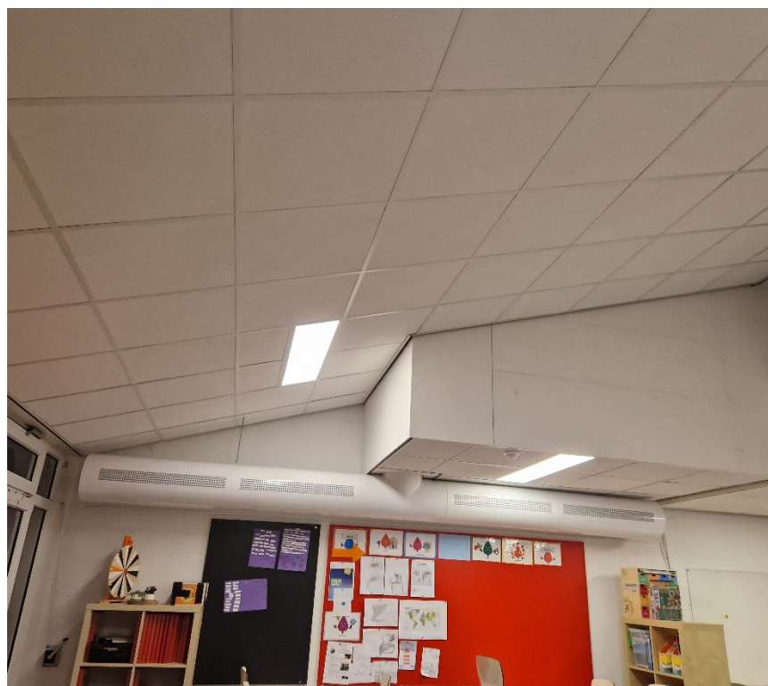
Figure 3-1 – Ventilation system after intervention C
