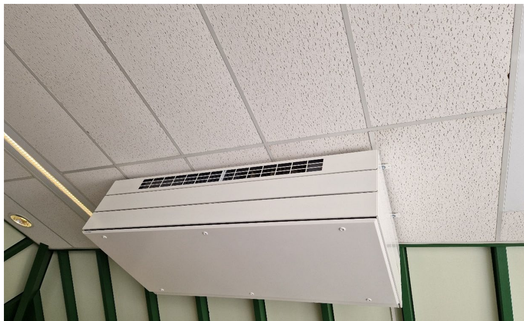
Figure 3-1 – Ventilation system after intervention
