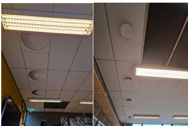
Figure 3-1 – Ventilation system after intervention
