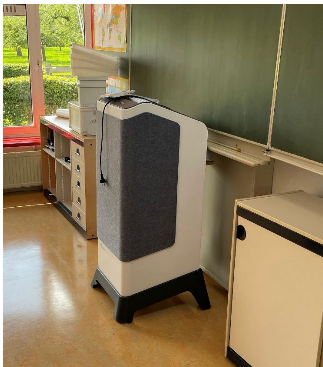
Figure 3-1 – Ventilation system after intervention
