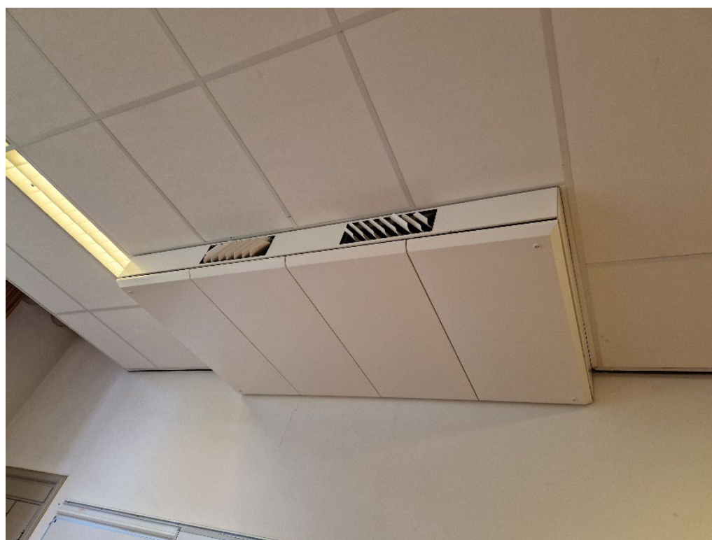
Figure 3-1 – Ventilation system after intervention
